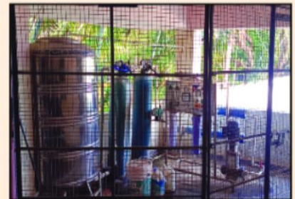
RO Water Plant Facility
