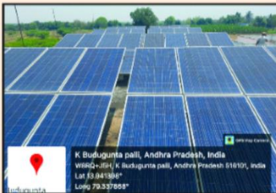
Solar Power Facility
